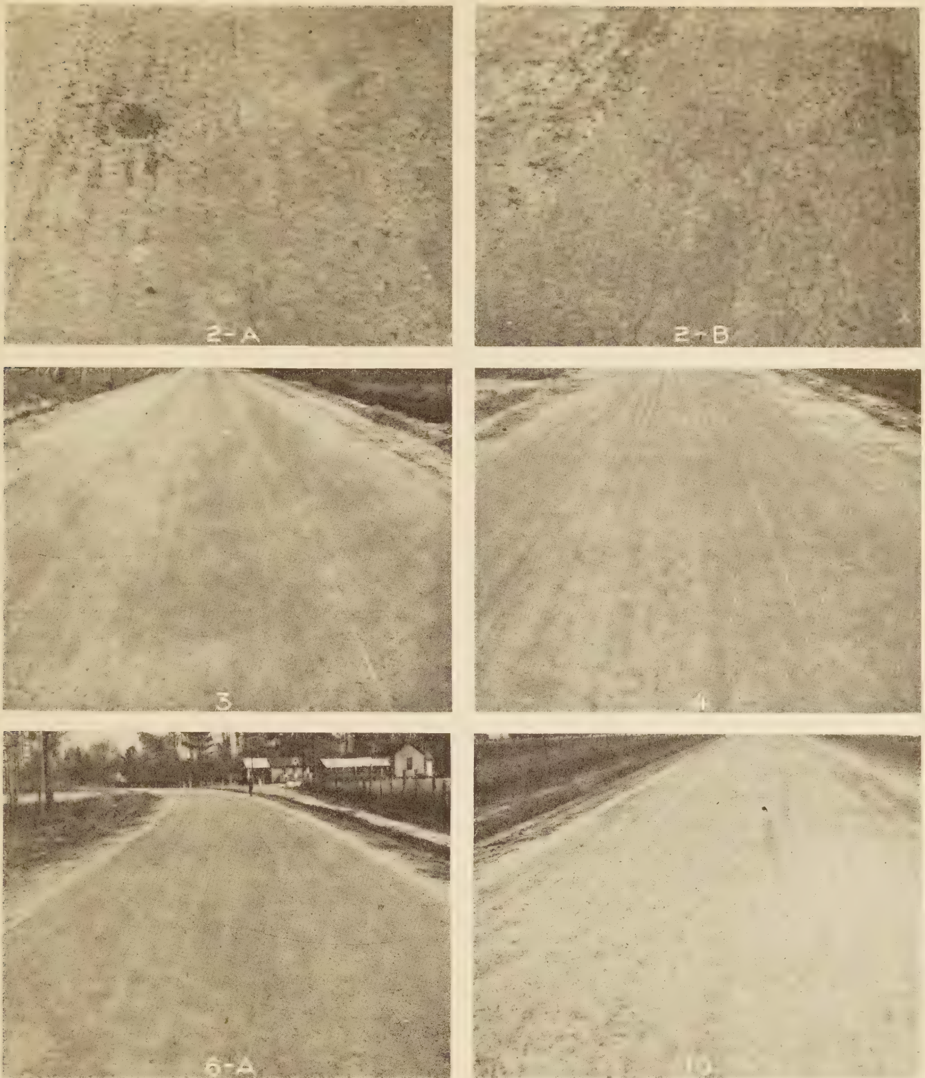
FIGURE 5.—EXAMPLES OF SURFACE APPEARANCE SIX MONTHS AFTER CONSTRUCTION. THE NUMBERS OF THE EXPERIMENTAL SECTIONS ARE GIVEN ON THE PHOTOGRAPHS. EXPERIMENTS 2-A AND 2-B: CRACKING AND RAVELING DURING SPRING OF 1930 WAS CAUSED BY SOFTENING OF THE MARL BASE AS A RESULT OF MOISTURE. EXPERIMENT 3: SECTION IN EXCELLENT CONDITION; MARL BASE, WHILE SLIGHTLY DAMP, HAD NOT SOFTENED AS IN EXPERIMENTS 2-A AND 2-B. EXPERIMENT 4: SURFACE IN GOOD CONDITION, EXCEPT FOR A FEW SMALL AREAS WHERE MARL BASE HAS SOFTENED. EXPERIMENT 6-A: IN EXCELLENT CONDITION; SAND-CLAY BASE MOIST, BUT ITS SUPPORTING VALUE APPARENTLY NOT AFFECTED. EXPERIMENT 10: GOOD CONDITION DUE TO EARLY RE-TREATMENT, WHICH NO DOUBT SAVED THE SECTION FROM COMPLETE DISINTEGRATION
